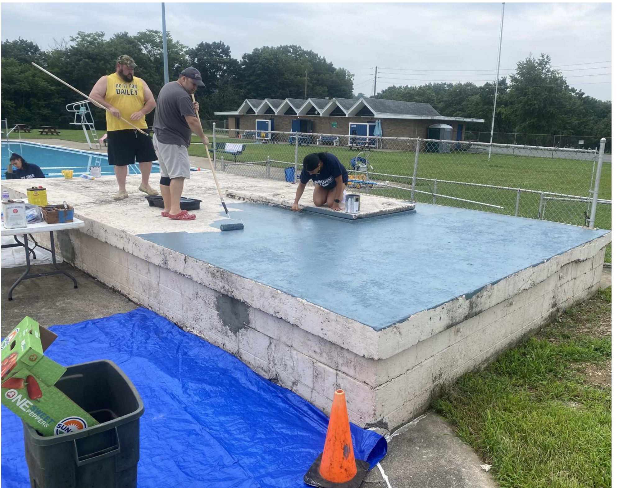
Mr. Tout, Mr. Sander, and Victoria Hanna paint the pool's chlorine house during the Nature Preservers' overhaul.
